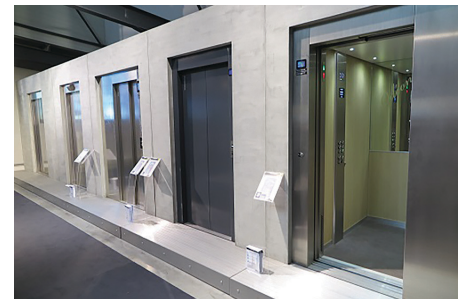
Sodimas designs custom high-end elevators that can be adapted to a wide variety of architectural styles and needs.
